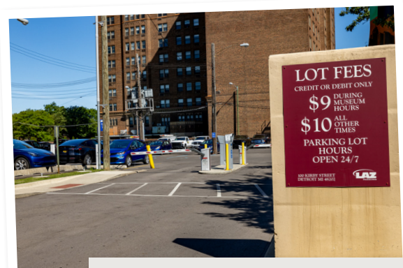
The Detroit Historical Museum's guest parking lot was completely repaired and repaved.
